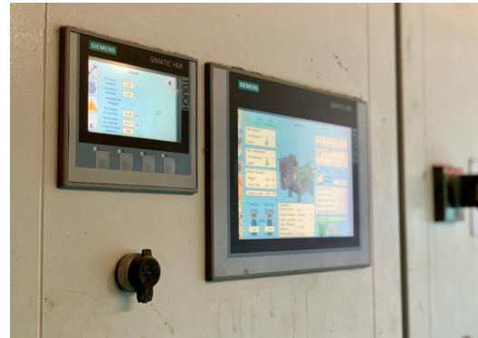
GHT decanter control panel
